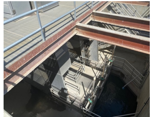
Taken at the NORSD waste-water treatment plant Photos courtesy of the Grand Jury
